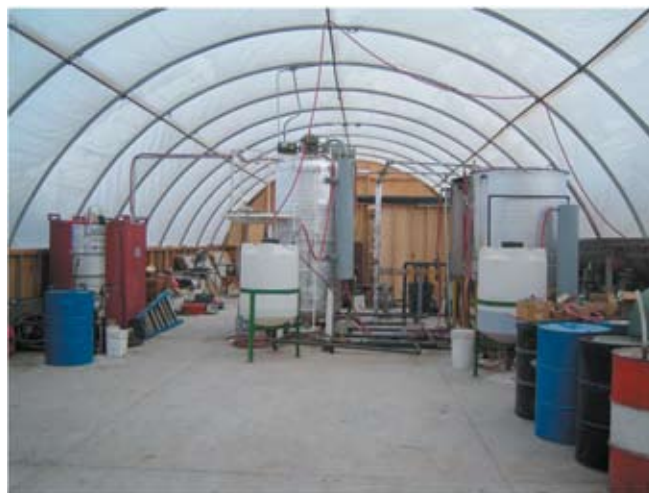
Figure 5. Photograph of the biodiesel production equipment.
