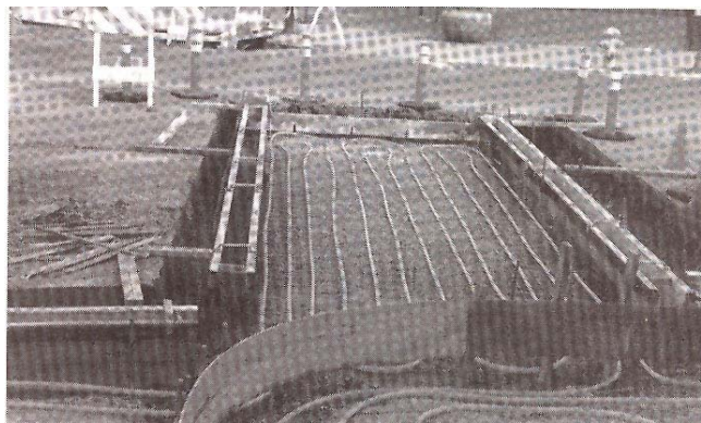
Figure 2. View of the tubing under a crosswalk.
