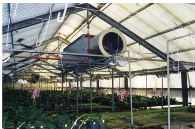
Figure 3. Forced air heat exchanger.
