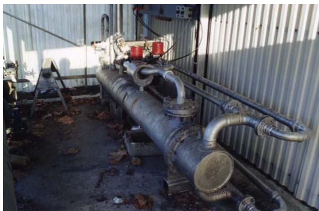
Figure 4. Main heat exchanger.
