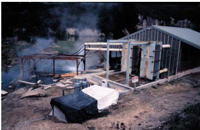
Figure 3. Hot water intake and plate heat exchanger.
