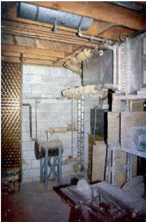
Figure 6. Heating system using forced air. DHE pipes enter at bottom right: forced-air heat exchanger at the top right (where a furnace used to be), expansion tank at top center, homemade shell-and-tube heat exchanger for the domestic hot water at the bottom center.
