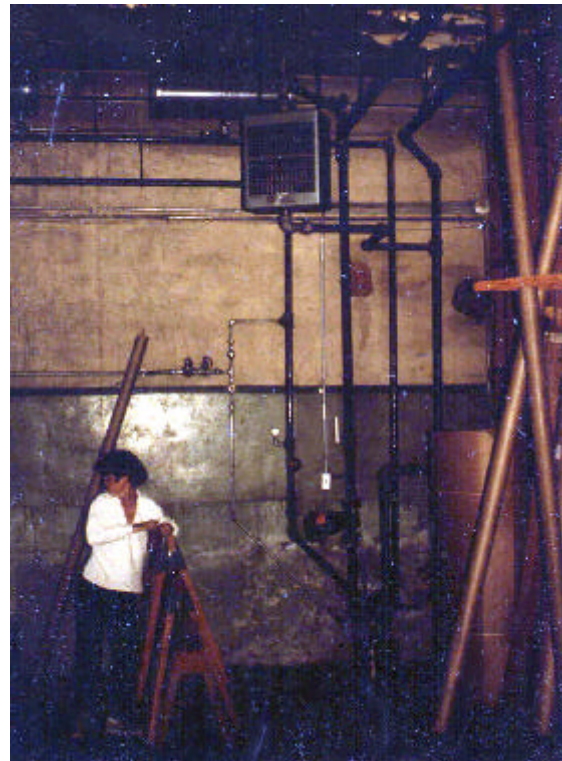
Figure 7. Commercial building heat system with two DHE heating loops entering the building at the bottom center; city secondary water entering through the pressure relief and pressure reducing valves on the left center; expansion tank at the upper center; and a finned-tubed unit heater at the top. The pipes run to other unit heaters throughout the building.
