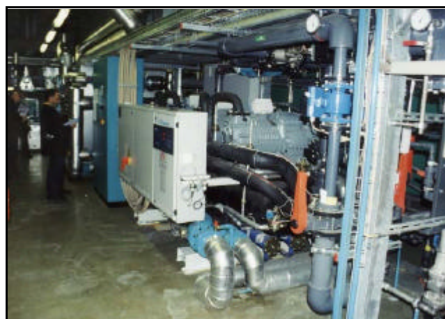
Figure 6. Heat pump equipment room.
