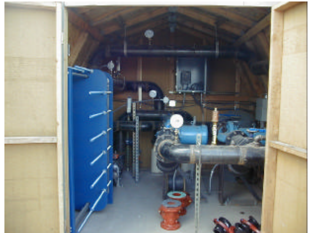
Figure 3. The main plate heat exchanger.
