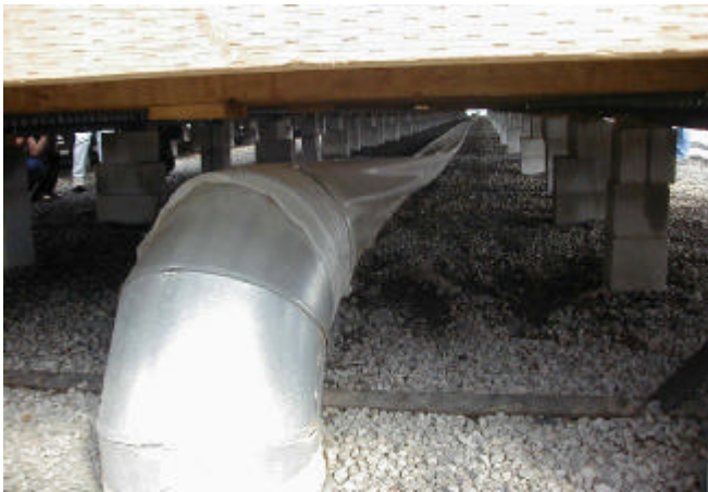
Figure 5. Under-bench heating system.
