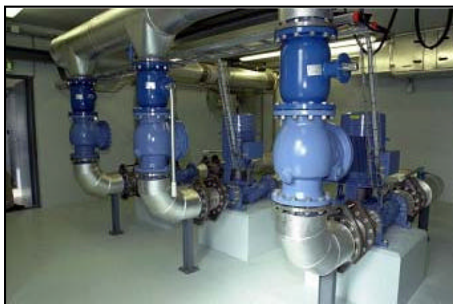
Figure 6. Inside the main pumping station.
