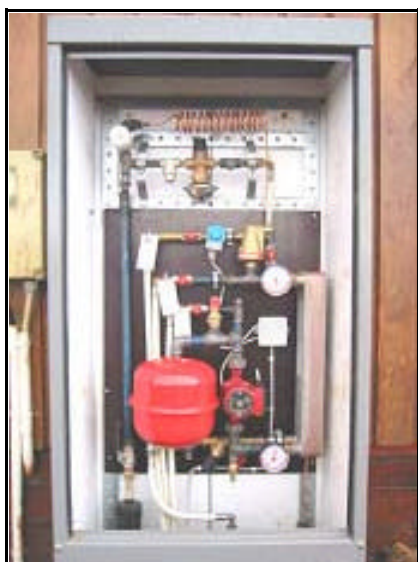
Figure 7. Geothermal connections in a country home cabinet.
