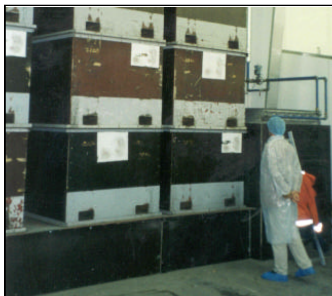
Photo 5. Secondary air-drying unit with geothermal pipes and controls on right.
