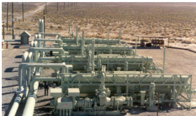
Figure 7. Binary power plant in Empire, Nevada.
