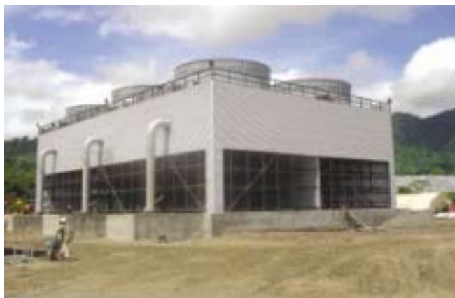
Figure 10: Lihir Back-Pressure Steam Power Station.
