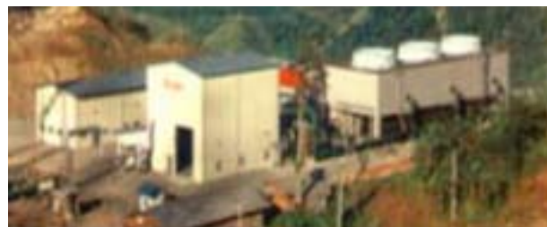
Figure 11: Leyte Binary Plant.
