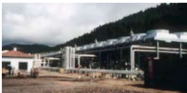
Figure 12: Ribeira Grande Binary Plant.
