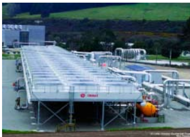
Figure 9: Wairakei Binary Plant.
