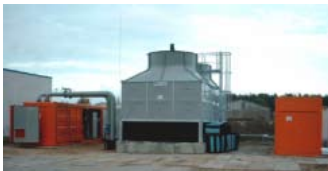
Figure 6: Neustadt Glewe Binary Plant.
