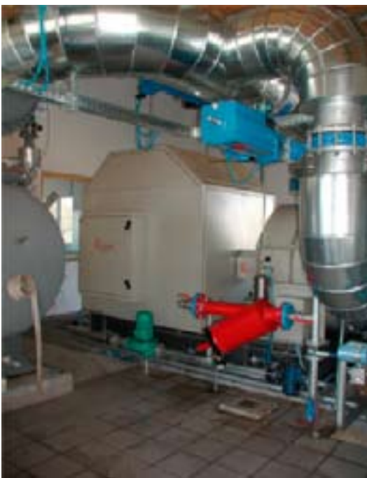
Figure 3: Altheim Binary Plant.
