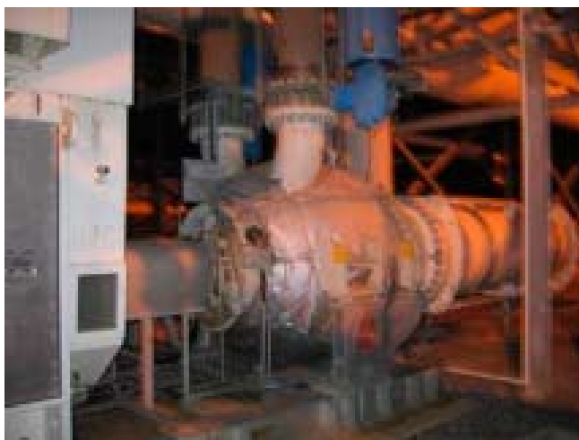
Figure 14: Salavatli Binary Plant.
